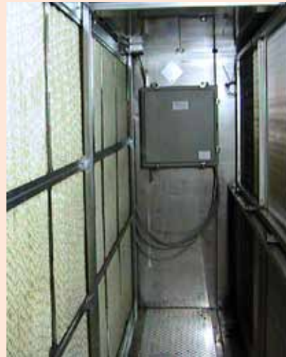
Trane Performance Climate Changer Field Retro-fit, Norman OK Library
