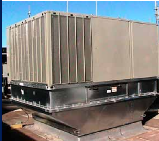
Norman Oklahoma Police Station RTU Change Out
