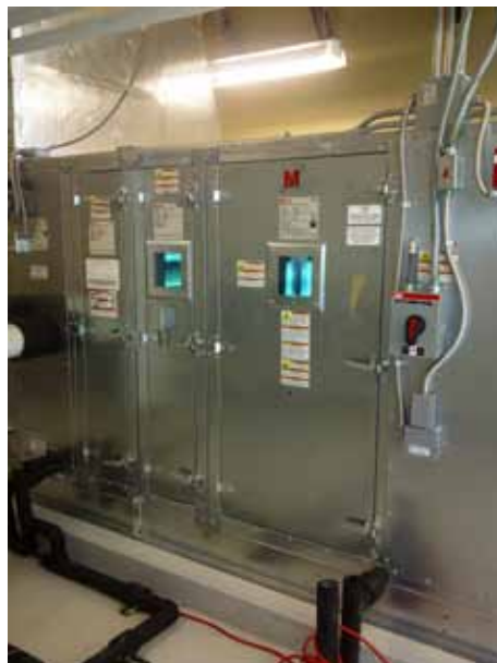
St Luke's Vintage Hospital TCACS Factory Install Houston, TX
