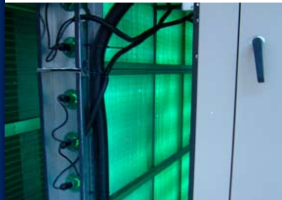
Typical PCP Standard install Fort Sam Houston
