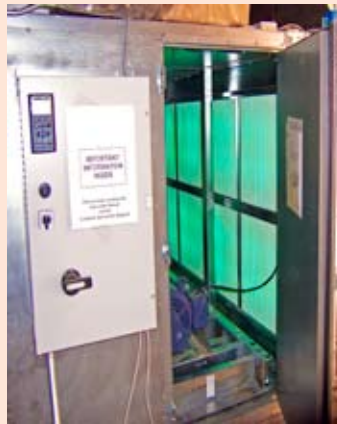
Trane Air Handler Homeland Security's FLETC Training Facility Artesia, New Mexico
